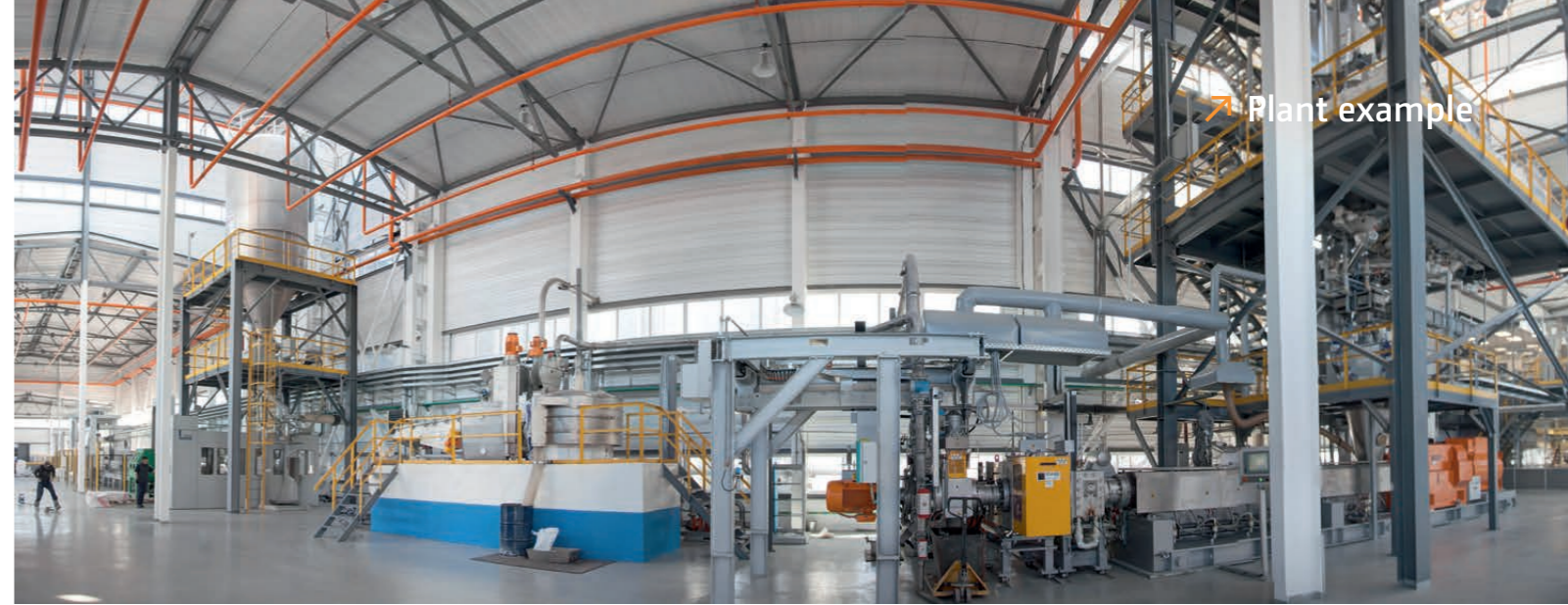
Panorama view of the overall plant
